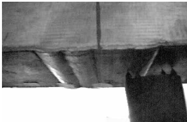
Figure 5.23 - The sensor is installed in the area of the fourth point
